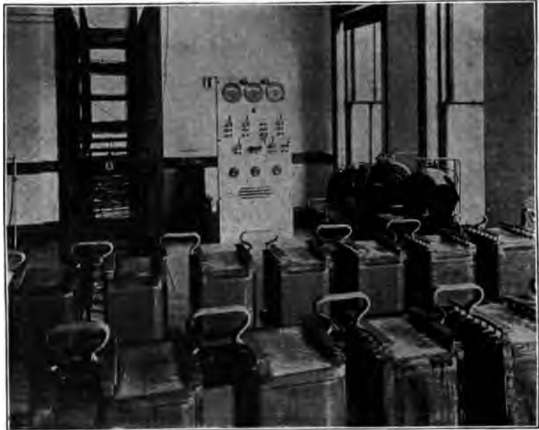
CORNER IN TELEPHONE EXCHANGE BATTERY ROOM. Showing power dynamos for connecting with 2,500 subscribers.
